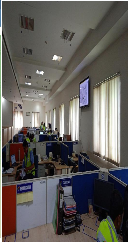
Scada monitor in CCR sitting area
